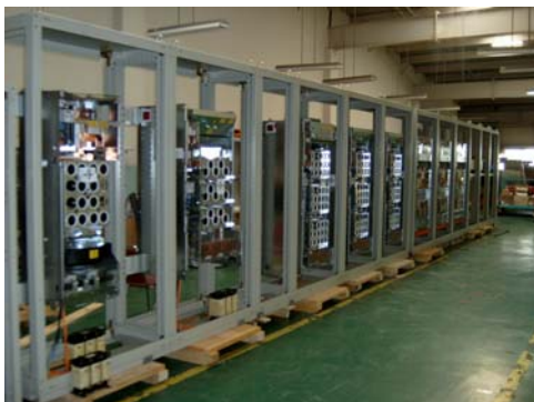
Drive and Inverter engineering and panel building
