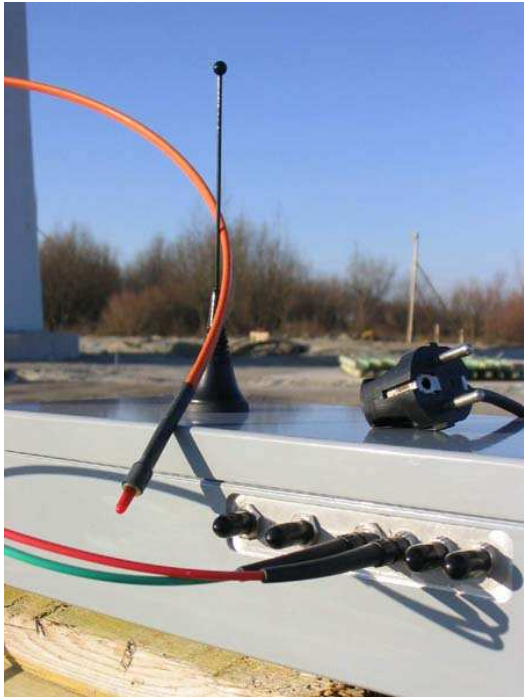
Control unit with sensor fiber
