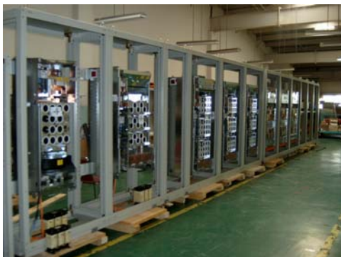
Drive and Inverter engineering and panel building
